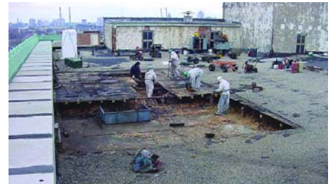
FJAC crews begin major demolition of old slope to drain wood structure.
